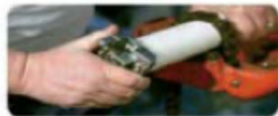
2. Pipe needs 10-15° chamfer (bevel). remove any dirt 管道倒角 10-15°, 清理边角碎屑
