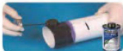
10. Apply a second application of cement to the pipe 胶粘剂再次涂抹管道
